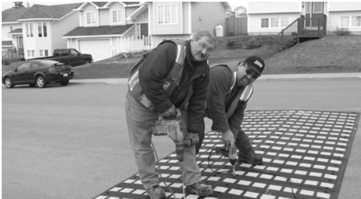
PUTTING DOWN THE SPEED BUMPS ----- Dean and Hugh Newman were busy Wednesday morning drilling holes into the pavement on Trails End in Paradise to secure the first of two new $6,000 speed bumps that will be installed there. The moveable speed bumps will be on this street for a while and then moved again to another spot in Paradise that has a bad reputation for speeding drivers. The holes they're drilling for the hardware to secure the speed bumps will stay in place and when, and if, the Town has to, they can put the bumps back into position in the future. These two workers with the Town of Paradise are not only colleagues, they're also brothers.
